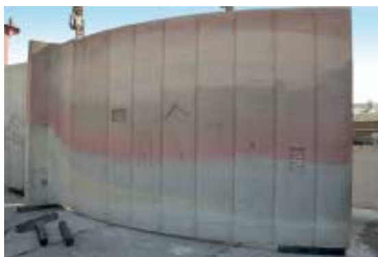
Fig. 7 For this curved wall, various concrete mixes and pigments were used to test different surface qualities and to make the flow behavior within the mold visible.
