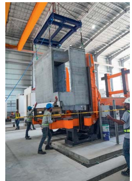
A suitable turning station was included in the equipment delivery
