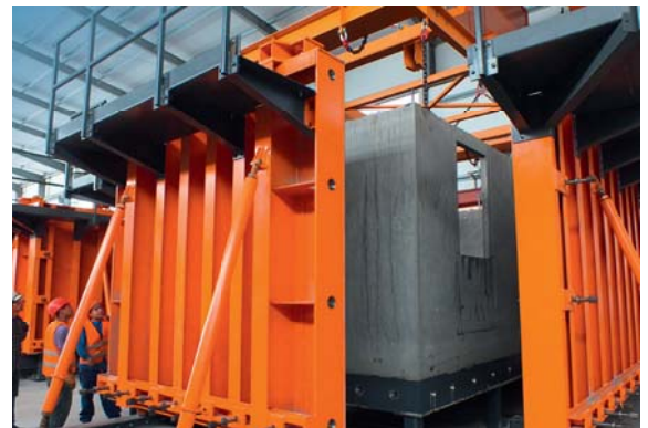
For production in installation position, the 35 t shrinking core is placed inside the mould for casting and lifted out for demoulding
