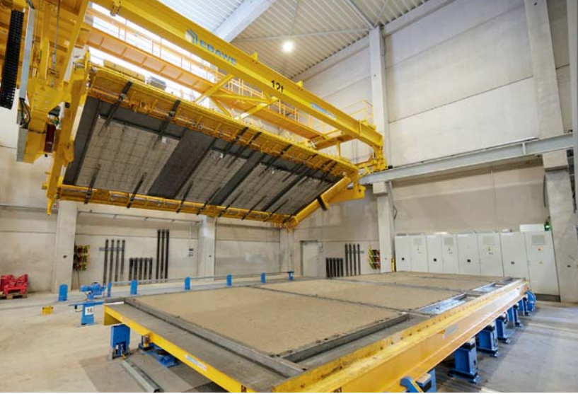
Turning device and clamping of the 1st shell for the double wall
